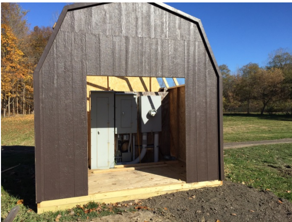
“Electrical building” at base of snow tubing hill.
