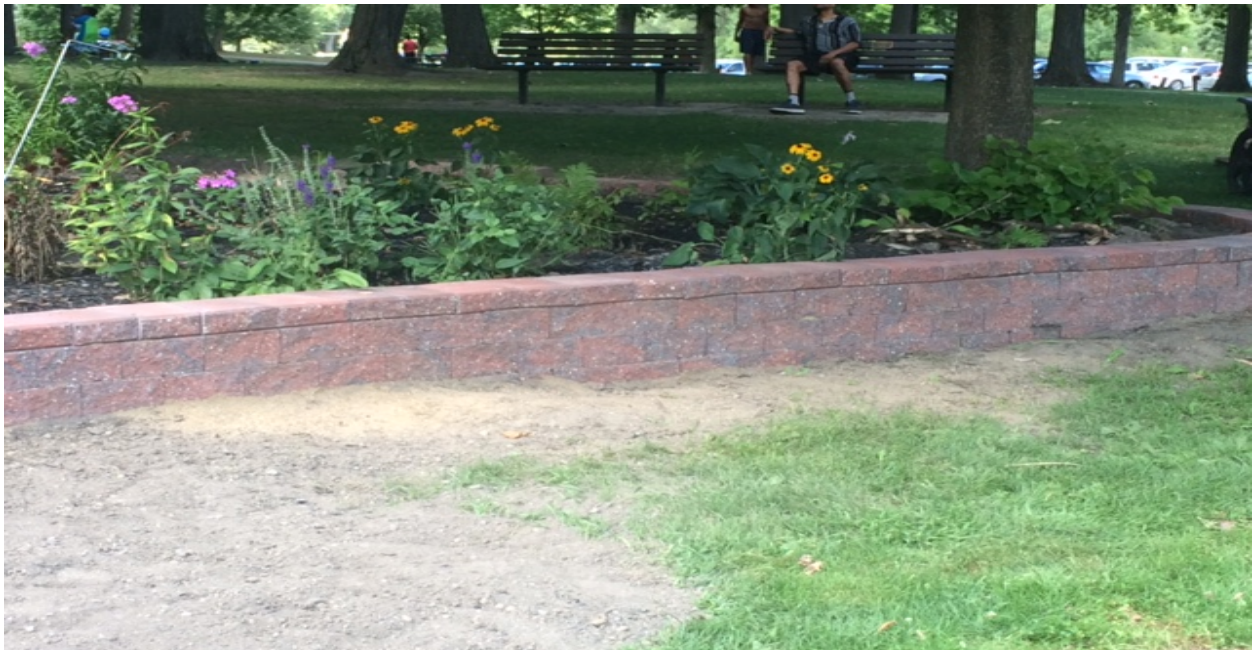
New retaining wall. Management Intern Travis Coon planned, researched, bid, and supervised a seasonal crew throughout the completion of this project.
