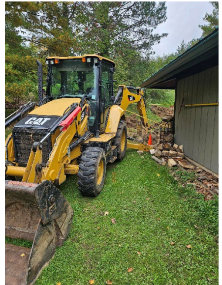
WSB Drain Line for Downspouts
