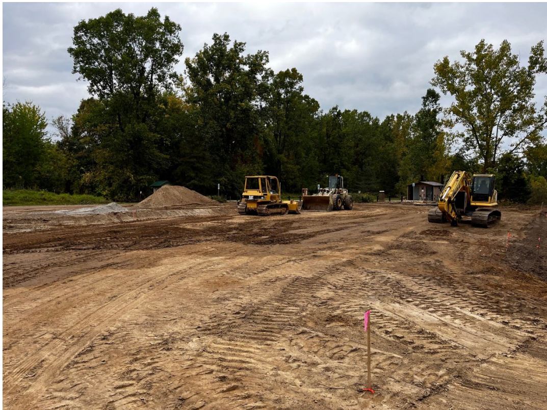
McNamara Landing parking lot progress prior to paving, hopefully w/o Oct 9th
